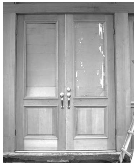
The new doors, moldings and columns of the old P.S. 17 building were painstakingly re-created under the supervision of United Homesteads, the contractor rebuilding the porch.
